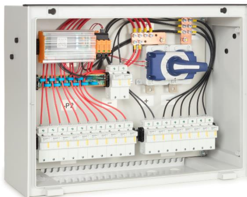
Image 3. Example of a combiner box with DAE equipped.
