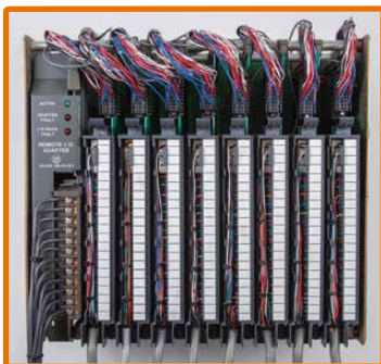
Completed and migrated PLC System
