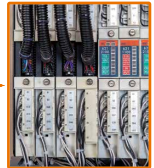
Completed and migrated DCS System
